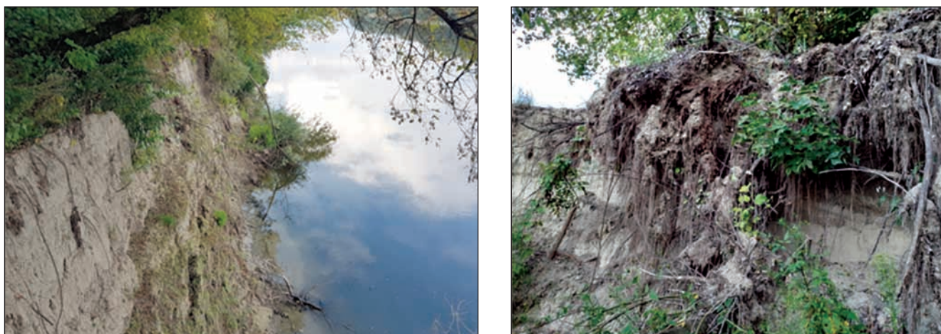
Fig. 16. Erosion of the land bridge downstream the bank protection area
