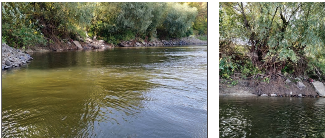
Fig. 15. Remains of bank protection with concrete slabs downstream the area of the stone facing
